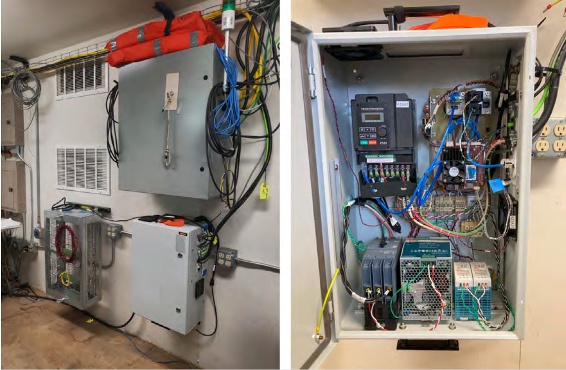
Figure 4: (left) The electronics enclosure and load dump installed in the lab on R/V Russell Davis Light . The AFT enclosure is the unit located lower on the wall. Cables exiting the electronics box are routed through the container walls to the gantry/frame where they are secured to AFT's support structures.
